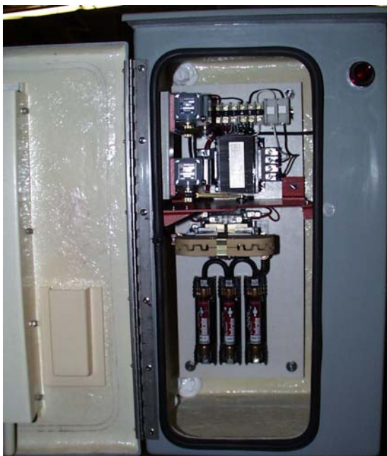
#050526 600 VDC Switch Heater Control Unit With 3 Load Fuses Used by CTA
